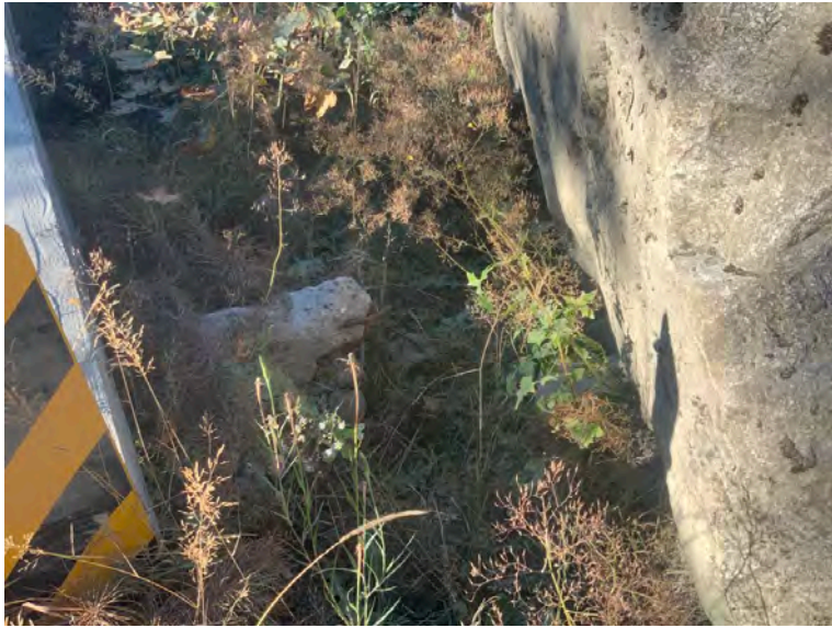
Ballast wall. Exposed rebar. Likely during install to fit around large rock
