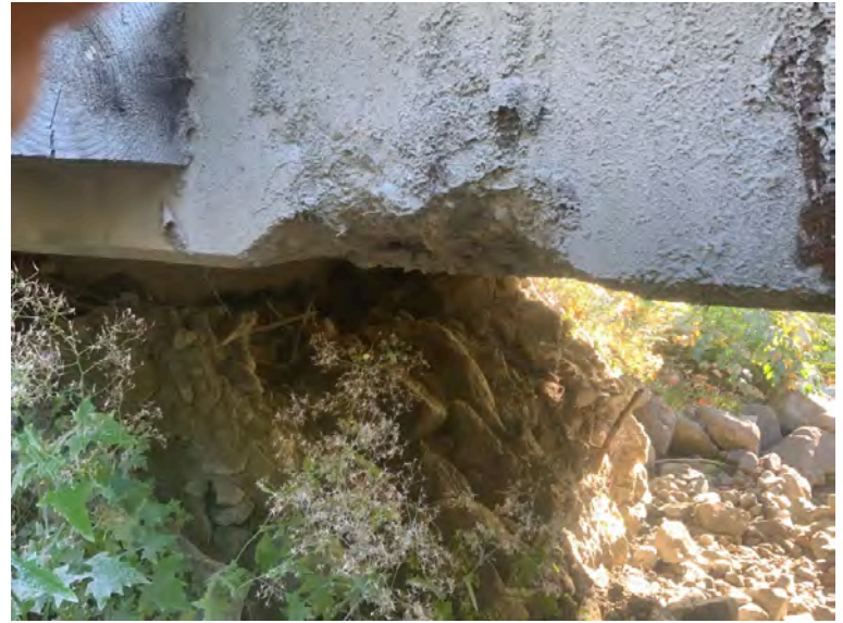
Slab damage. 40x10x15 cm. Exposed rebar
